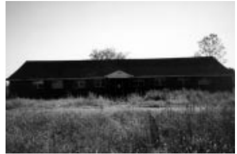
The Trades Building is in poor condition and should be demolished for safety. The bricks, however, could be salvaged and used by the future Job Training courses.
