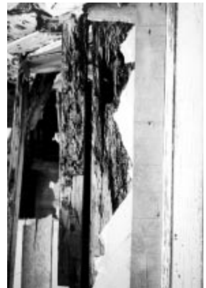
Decaying material found in one of the buildings
