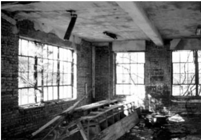
Materials may be stored in McDougall Hall, once all interior non-structural partitions are removed.
